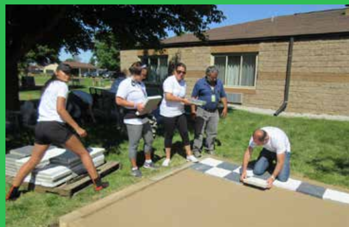
With oversight from HDC's Maintenance Supervisor Ed Gohn (blue shirt), folks from UBS carefully placed black and white blocks to form a checkerboard for the sensory path's outdoor games station.
